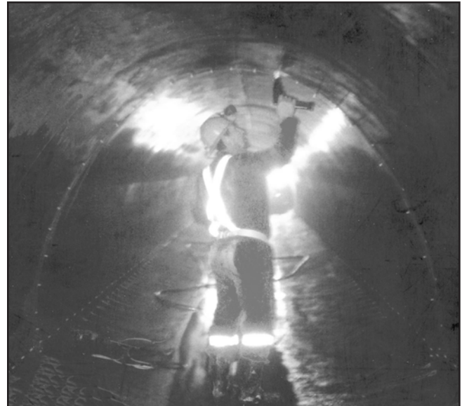
Cracks and joints in potable water structures such as the Shoal Lake Aqueduct are sealed with FLEXIBLE resin
