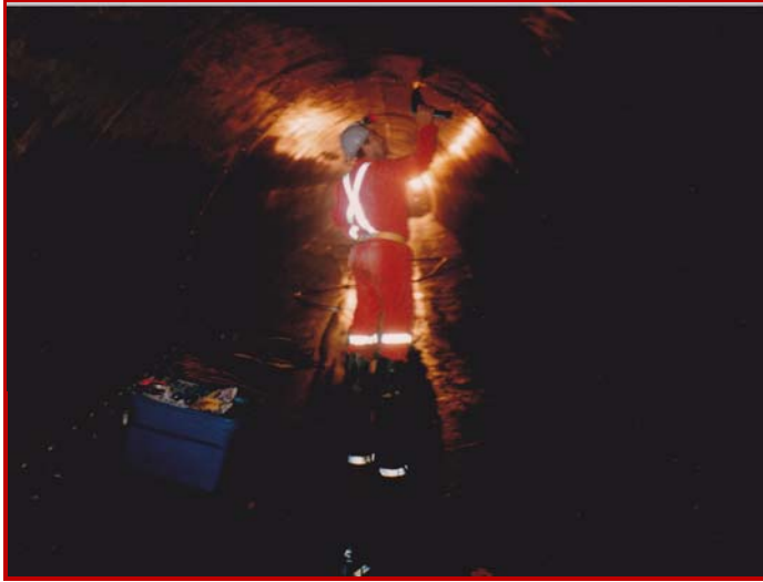
Cracks and construction joints in potable water structures are permanently sealed with FLEXIBLE RESIN.
