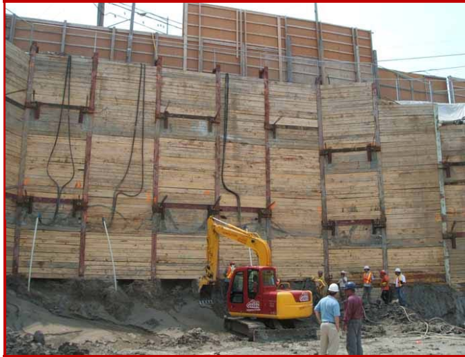
Soil liquefaction problems at a deep excavation site were overcome using ULTRAFINE RESIN; A fast-curing, hydrophobic polyurethane.
