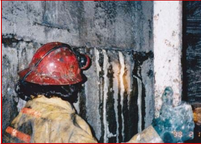
UNIVERSAL RESIN is used to stop water inflows through leaking concrete construction joints in an underground mine shaft.
