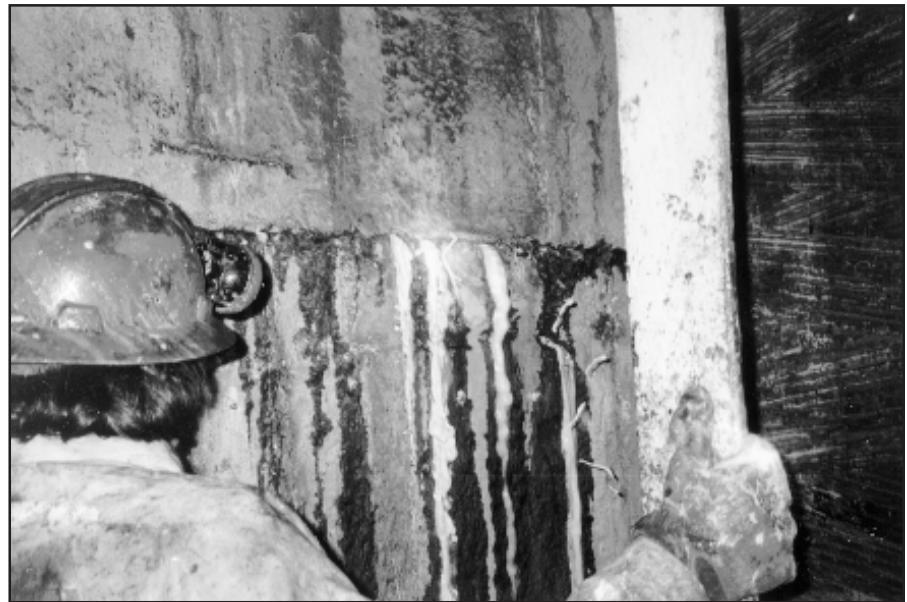
Water-activated polyurethane foam used to stop water inflows through leaking concrete construction joints in underground mine shaft lining using UNIVERSAL resin
