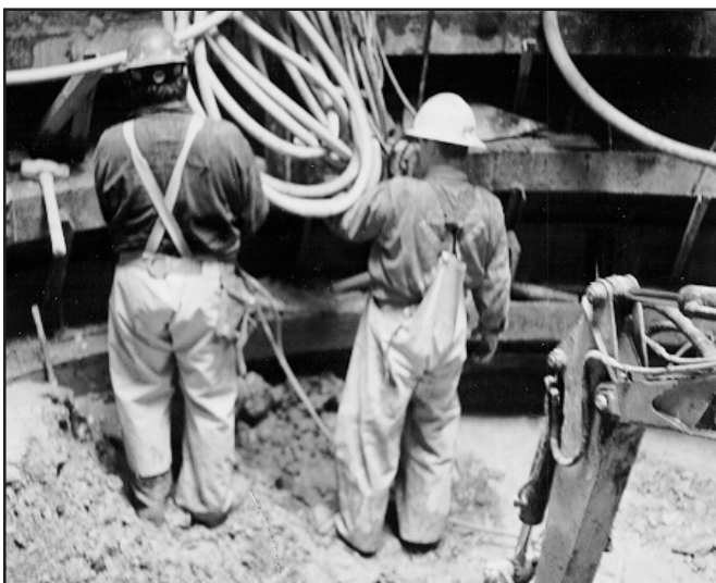
Miners preparing for polyurethane injection to stop inflows of quicksand into a 24 foot diameter shaft collar excavation
