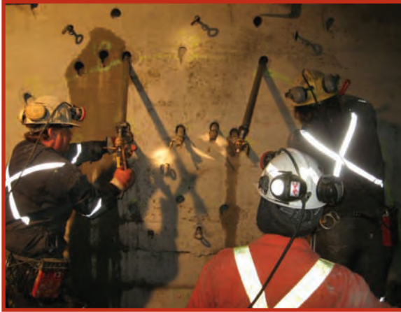
Hudbay Minerals, 777 Mine, Manitoba Specialized grouting equipment and technical support was used in the construction of two high-pressure concrete bulkheads.
