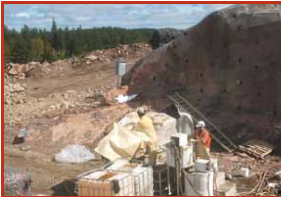
FNX Mining, Podolsky Mine, Ontario Pre-grouting of raise bore holes was completed using microfine cement grouts, equipment and technical support.
