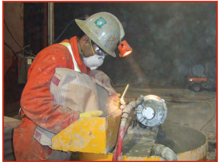
Sifto Salt, Goderich Mine, Ontario Chemical grout, applied as spray foam, was used to seal a five meter high by eight meter wide underground ventilation bulkhead. A layer of cement grout (in the form of spray foam) was applied over top for fire protection purposes.
