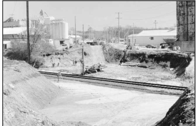
A large soil stabilization project was undertaken to allow bridge reconstruction on unstable ground beneath an active railway line adjacent to an operating limestone plant based on engineering recommendations from technical specialists of MULTIURETHANES
