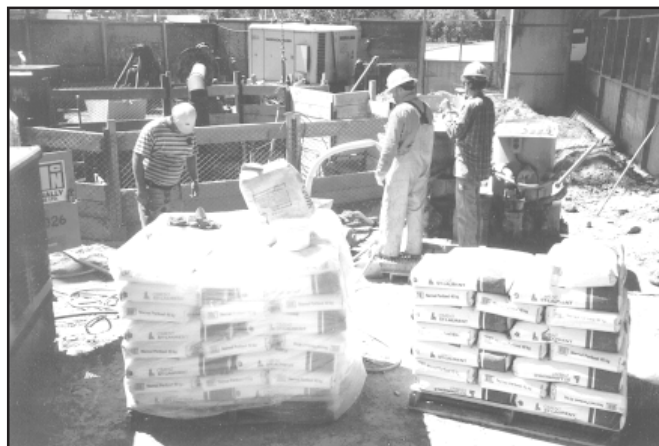
Cement grouting operation where colloidal mixers were used to prepare stable, balanced cement grout containing bentonite and superplasticizer additives for stabilizing loose, water-bearing soil adjacent to sheet pile wall surrounding vertical shaft; technical supervision by grouting specialist from MULTIURETHANES
