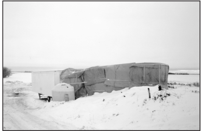
At this cold weather job site, grouting crews were protected from the elements utilizing heated vans and tarps
