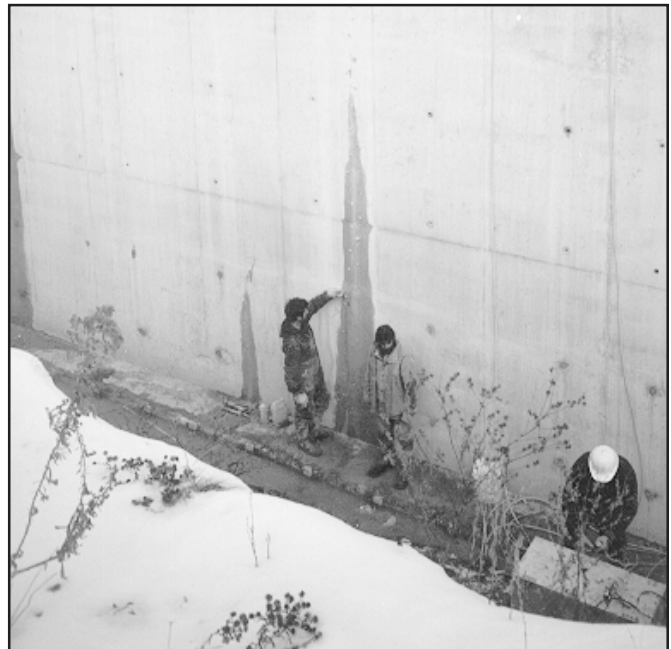
Crews at this potable water reservoir used electric pail heaters to maintain flushing solutions and polyurethane resins at elevated temperatures to combat sub-freezing temperature conditions
