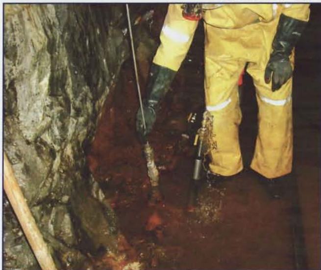
Experienced grouting technicians work together to stop the most difficult water flows.
