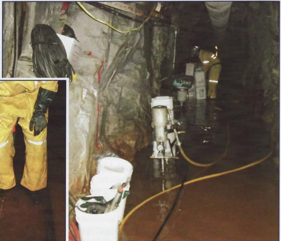
From high volume flowing water to a dry tunnel. Call Multiurethanes when difficult ground conditions are experienced on your jobsite.
